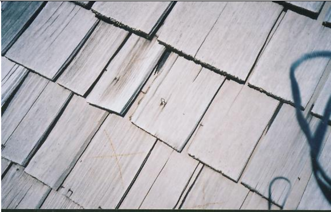
Shake shingle burn-out
