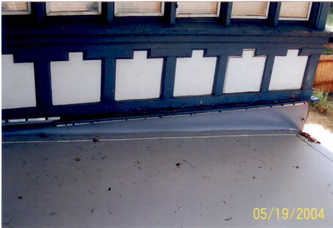
Picture #6 We frequently use colored TPO on flatroofs with overlooking windows. This way nobody looking out a window gets blinded by reflecting sunlight.
