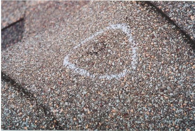
Hail often damages ridge shingles.
