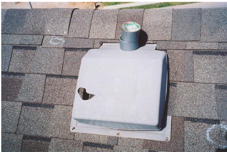
Hail hits can leave large leak-prone holes in vents. Duct tape can provide a quick emergency repair.
