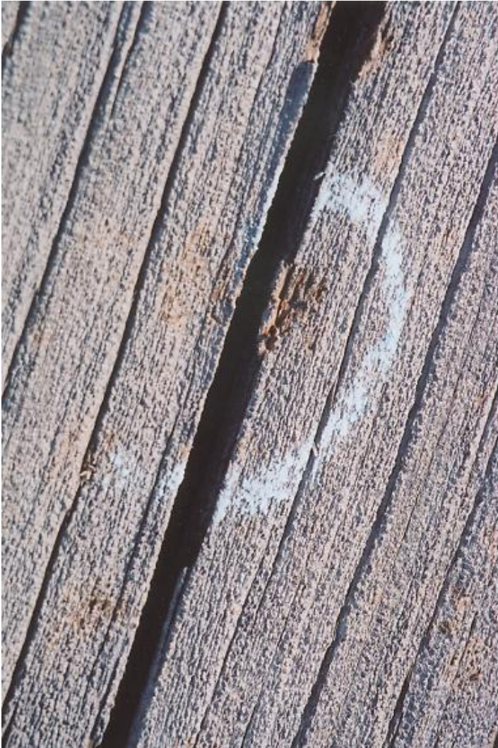
Photo #10 This hit qualifies for HAAG because fresh wood is exposed.
