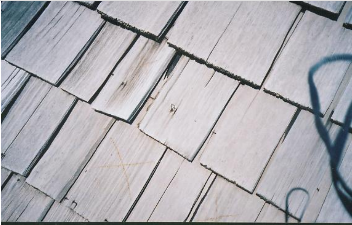
Shake shingle burn-out
